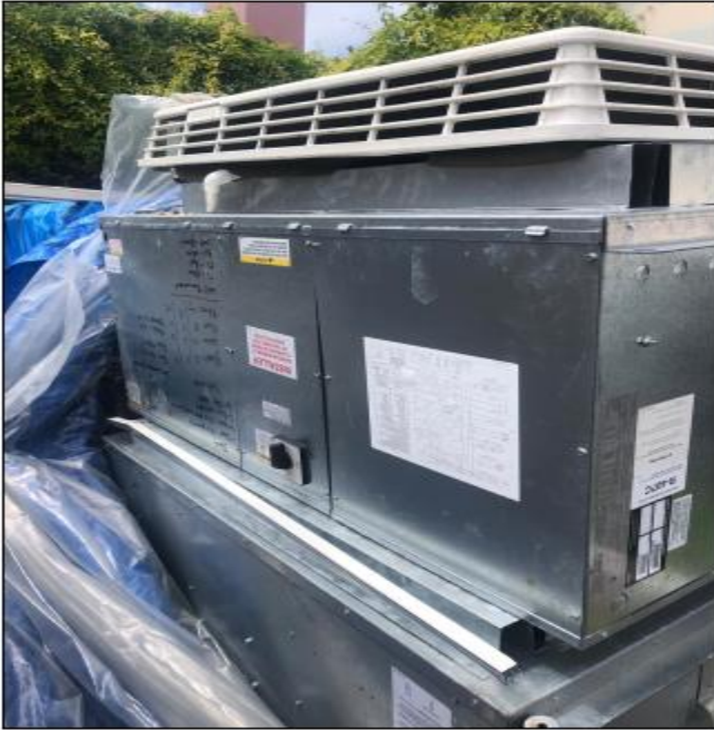
1) Air Handler Unit (3 ton)
