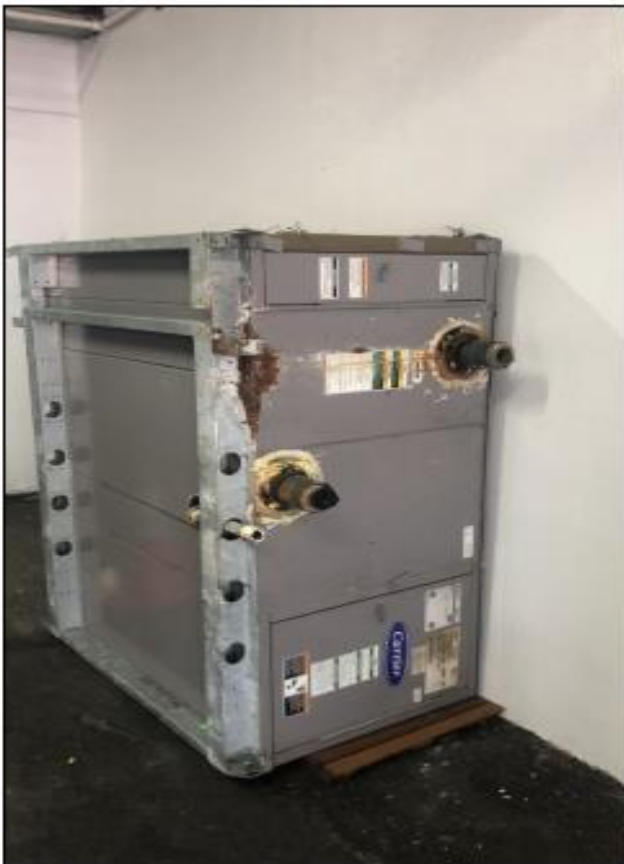
2) Chilled Water Air Handler (8 ton)
