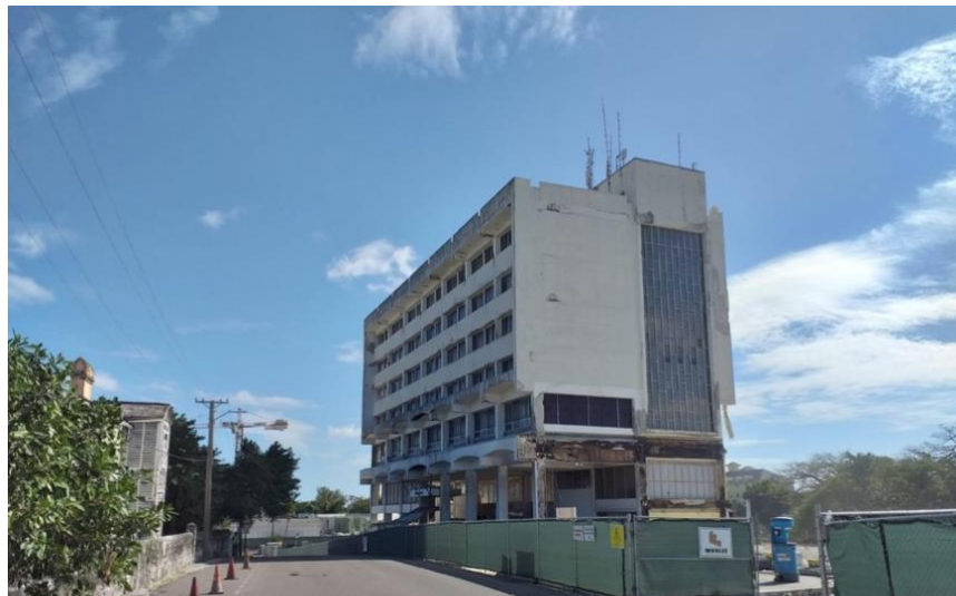
Post Office building during demolition (2021). View looking east from East Hill Street.
