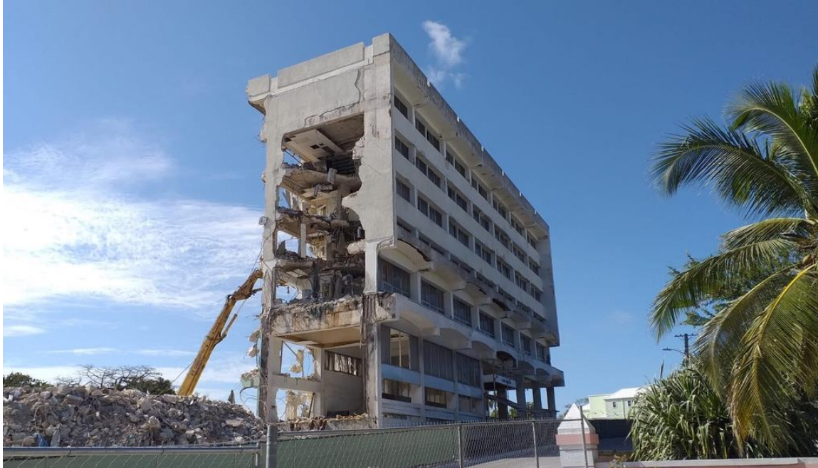
Post Office building during demolition (2021). View looking west from East Hill Street.
